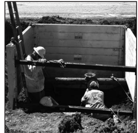
Three-sided configuration with spreaders on long side and removed bottom panels to straddle pipe
