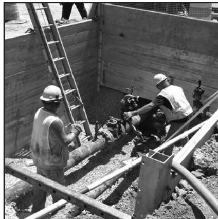
A three-sided configuration with end panels pinned 1 ft. up in corner posts allowing gas utility to run through
