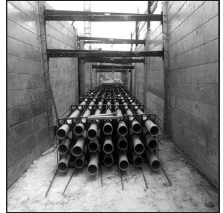
A series of two-sided configured Build-A-Box shielding a long pipeline
